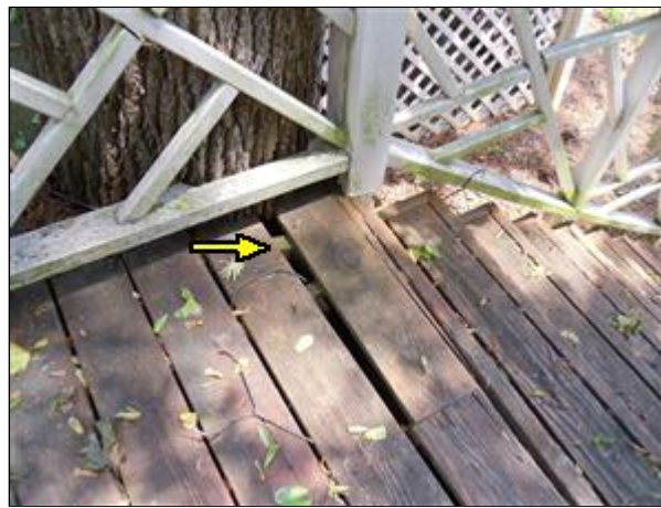
2.4 Picture 6 tree causing damage
