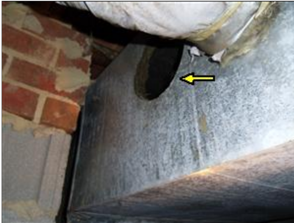
6.3 Picture 1 open supply hole
