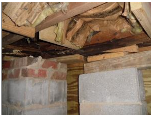
1.1 Picture 2 deterioration behind shower
