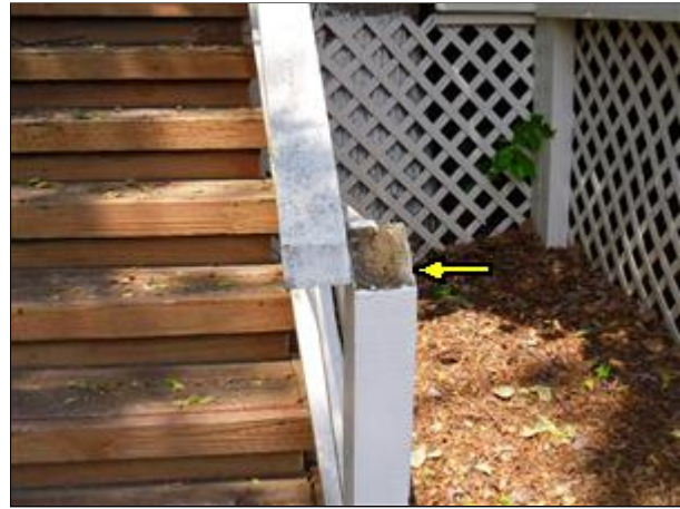
2.4 Picture 5 damage hand rail at back deck
