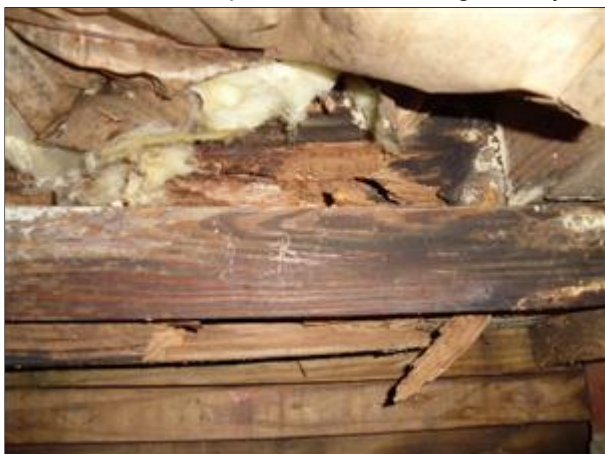
1.1 Picture 1 deteriorated outer band and sill
