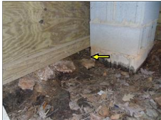
1.0 Picture 4 hole at right rear corner
