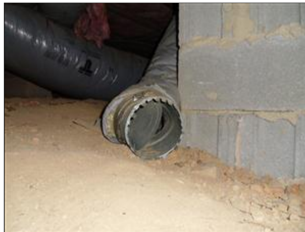
6.3 Picture 3 disconnected supply duct
