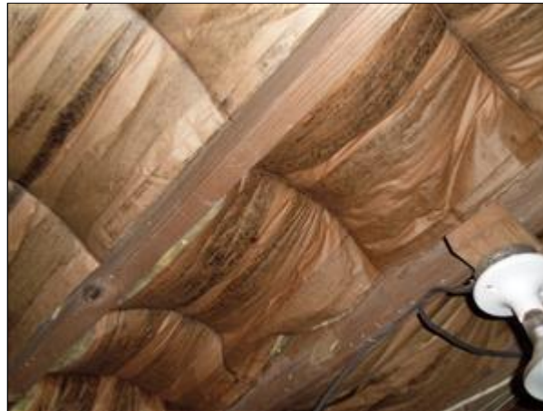
9.1 Picture 1 insulation upside down
